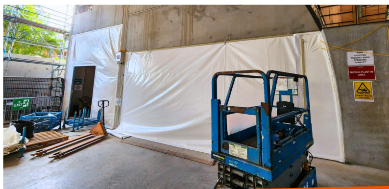
Roll-up Tuffclad Curtains with Rope Pulley System
